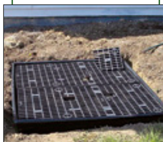
D. Cut holes in grating and mesh for fountain tubing and pump access.
